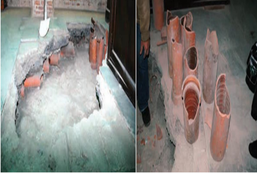
Figure 8. Clay pots used in the flooring system of the Hazine-i Evrak Building in Constantinople. Source: Atay, Gül (2021, 1–12, on p. 8).
